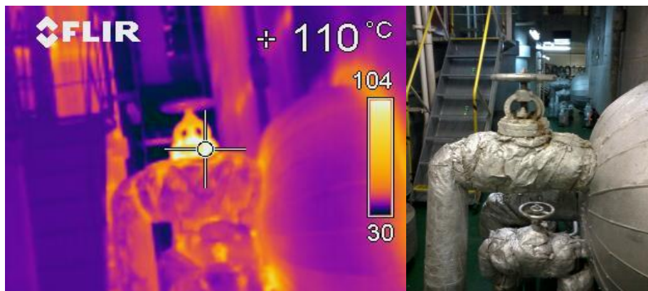
Fig. 2: Boiler's Steam Line.
