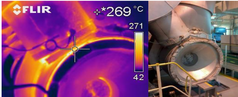
Fig. 1: Exhaust Gas Outlet of M/E to T/C No.1
